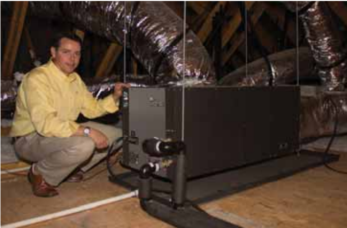
ClimateMaster Builder Development Manager Titian Burris kneels beside a ClimateMaster Geothermal Heat Pump in a home attic in Somer's Pointe.
