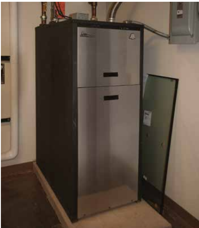
TMW unit in the mechanical room off of the cafeteria provides heating and cooling, plus hot water.
