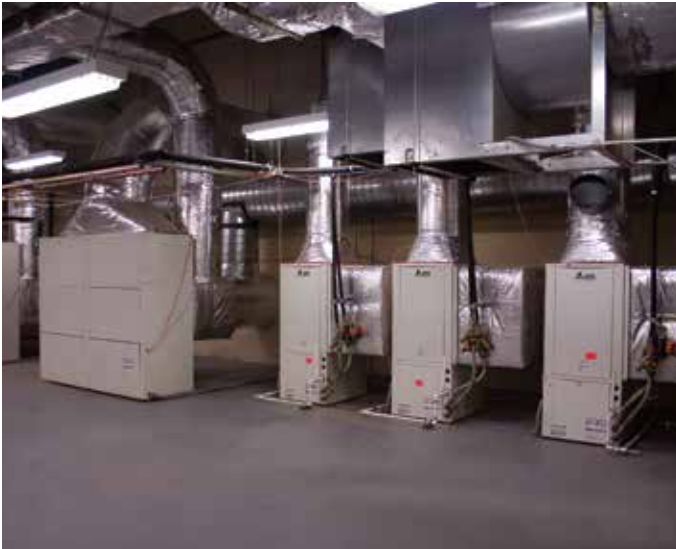
ClimateMaster heat pumps at work in Western Heights Middle School
