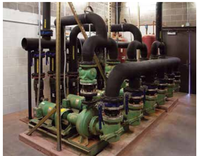
The pump room at Western Heights Middle School
