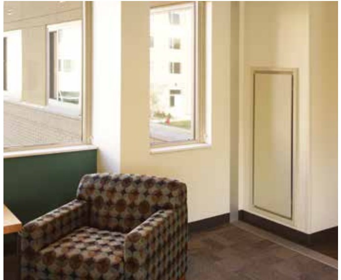
Tranquility Vertical Stack (TRM) units installed in Centennial Hall were finished with attractive return air panels
