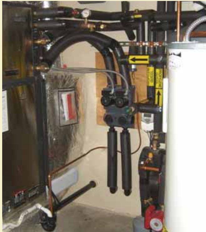
ClimateMaster 5 ton Tranquility 27 geothermal heat pump system.
